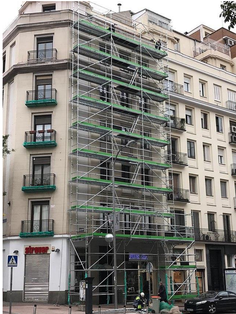
Scaffolding tied to building – This is not an example of a self-supporting structure because the building adds stability to the scaffold.
