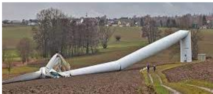
Buckling of a wind turbine
